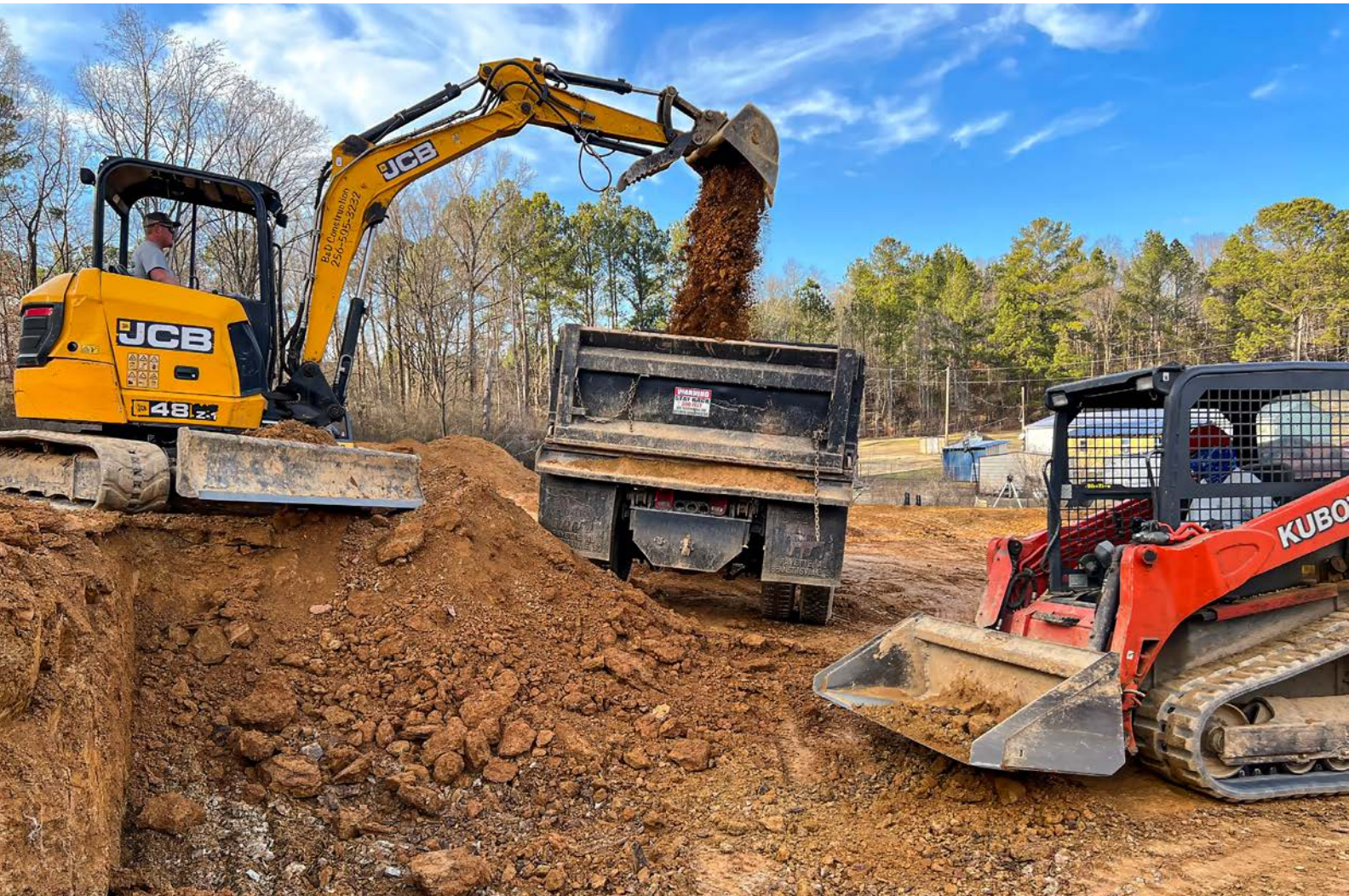
Dirt and crew members of the B&D Construction team on what has become a regular day of work
